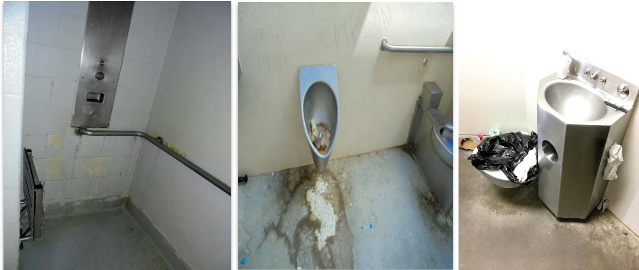
Figure 4. Shower stall with mold, mildew, and peeling paint (left). Outdoor recreation area with stuffed and overflowing toilet (center). Observed by OIG at the Adelanto facility on May 1, 2018. Detainee bathroom with mold and non-working toilet (right). Observed by OIG at the Essex facility on July 24, 2018. Source: OIG
